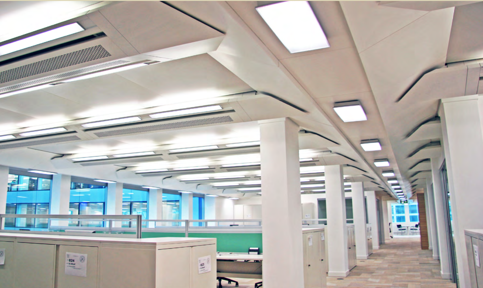
55 Baker Street original installation - 2007
