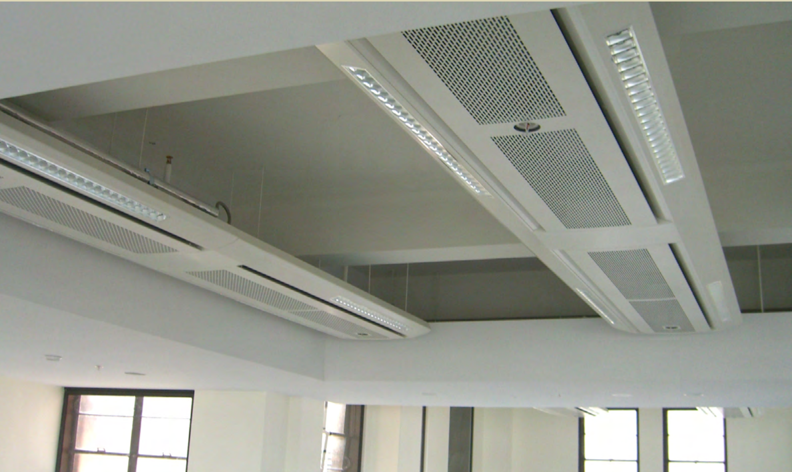
Transport House original installation - 2008
