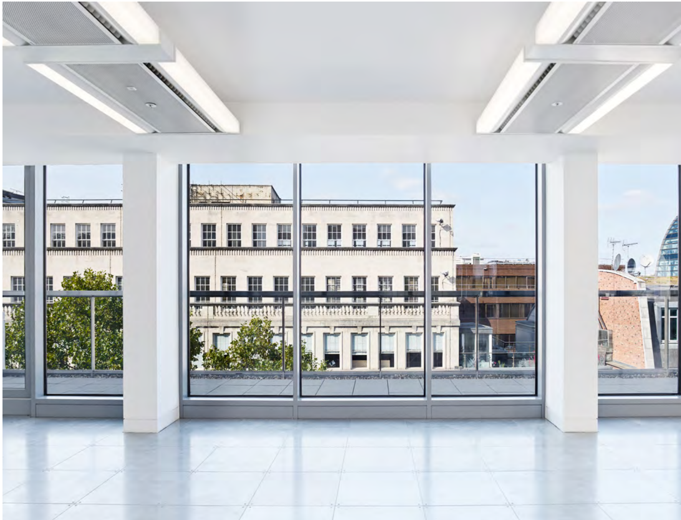
active multiservice chilled beams
