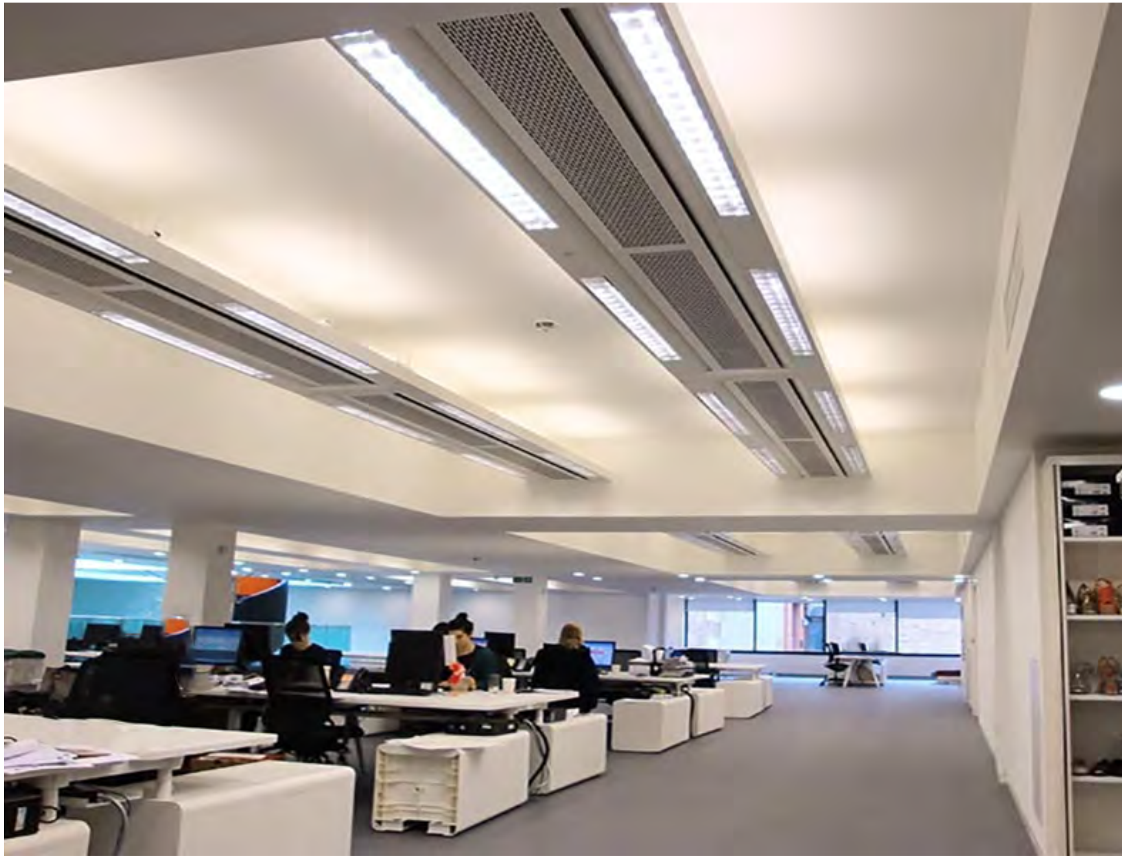
active chilled beams
