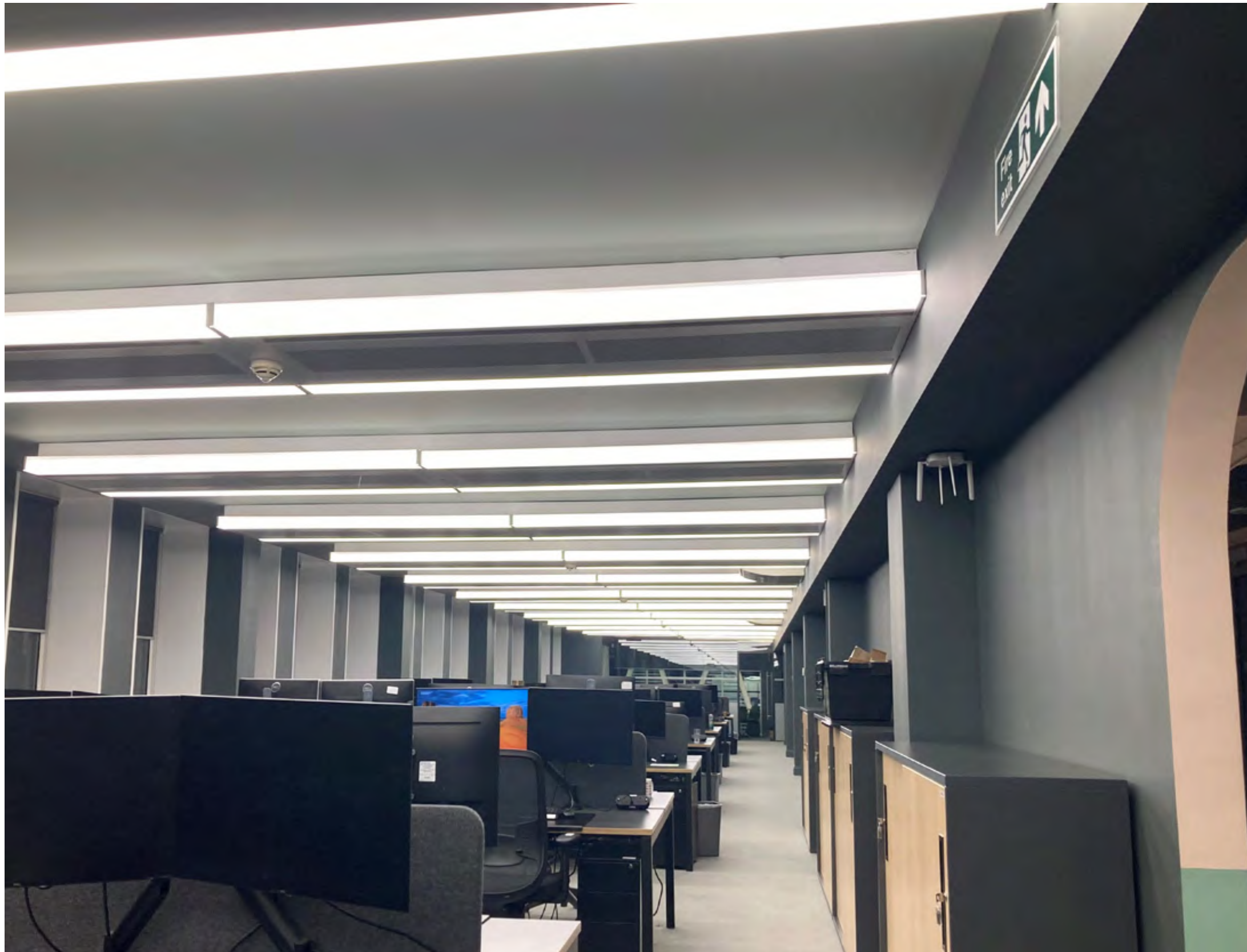
active multiservice chilled beams
