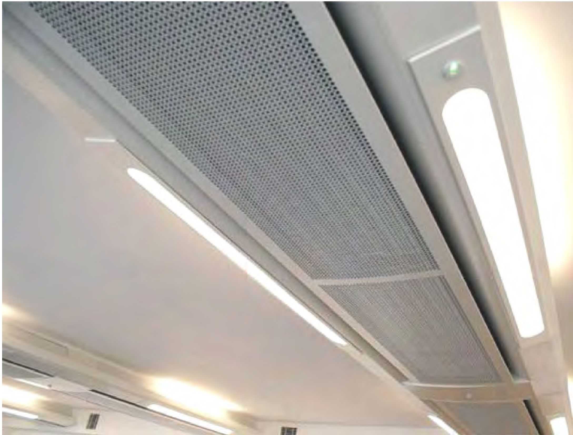
active multiservice chilled beams
