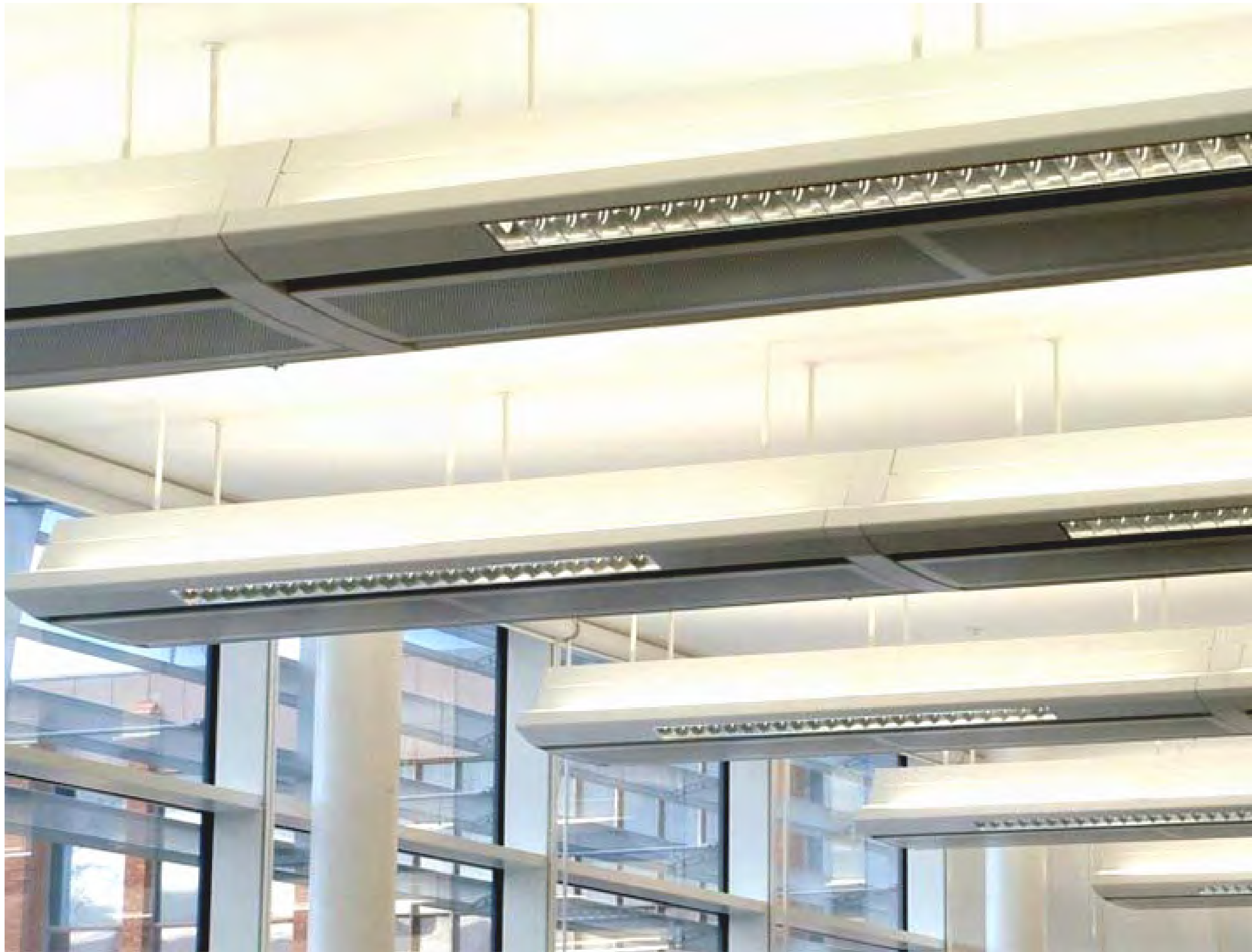
active multiservice chilled beams
