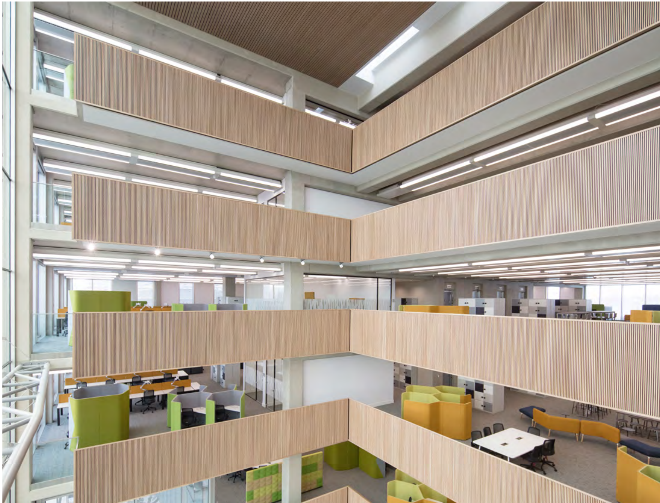
active multiservice chilled beams
