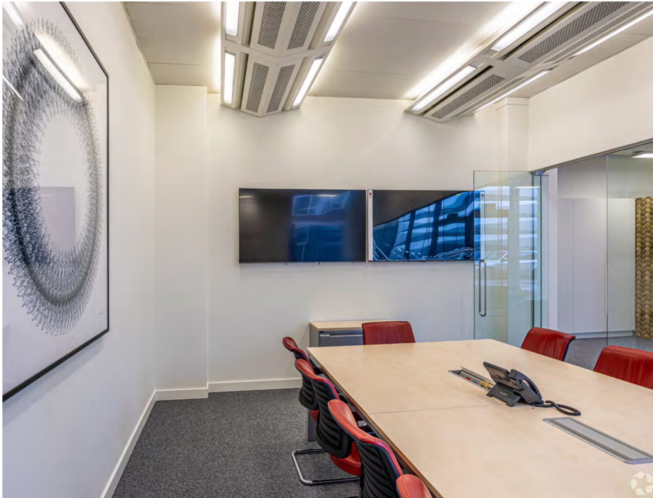
active multiservice chilled beams
